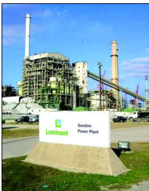
ABOVE: The Sandow 4 unit under construction in 1979 near Rockdale in southern Milam County. The plant originated to generate electricity for Alcoa's Rockdale Operations smelter.
